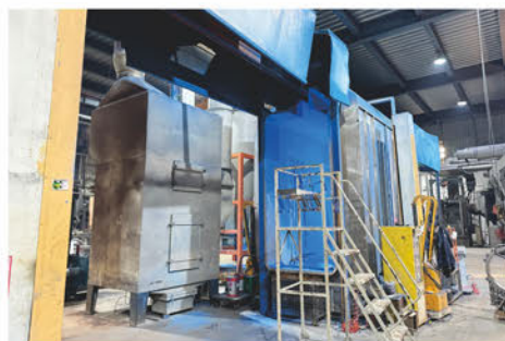
DN600-3M 静电喷涂流水线 DN600-3M Electrostatic spraying line
